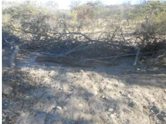
The repaired and fortified narrow breach in the top filter that had a domino affect on the two lower filters
